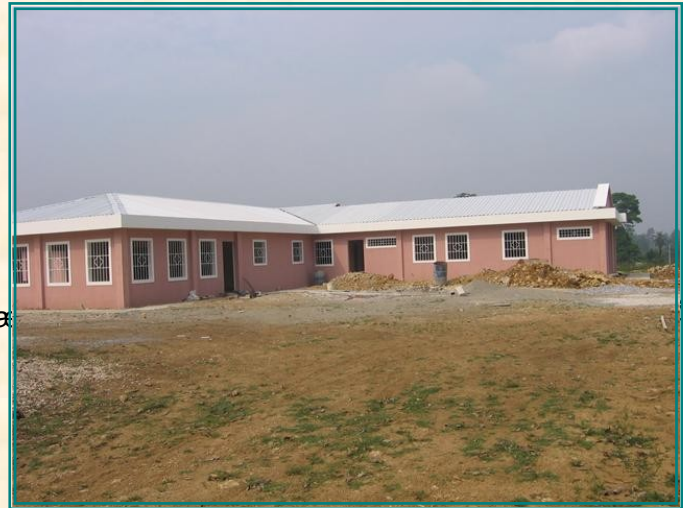
The new Medical Dental Clinic in Machaquila, ready to be finished need of windows and doors.
